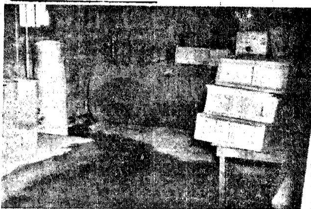
STORAGE ROOM — The storage room of the Riverside School is practically a running spring. The room has about two or three inches of water standing most all time. This leads to a poor health condition in the school. The tank in the corner is the water supply for the school. Anything that the teachers have to store must be placed on the table to the right of the picture.
